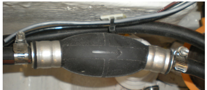
FUEL PRIMER BULB IN SUMP AREA
