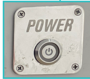
Battery activation panel
