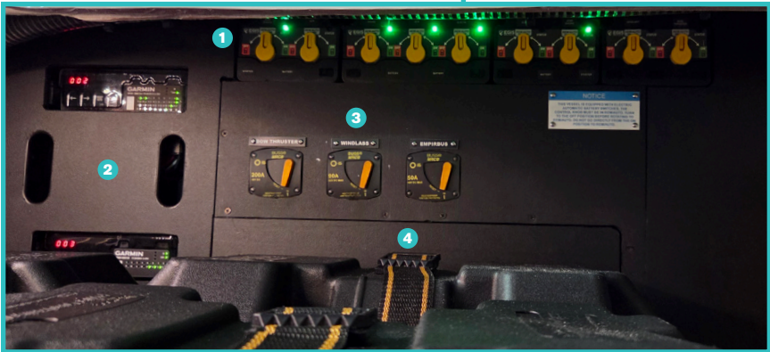
Battery management box
