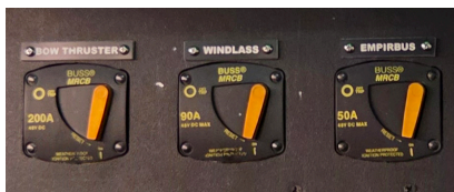
Dedicated high-amp breaker switches
