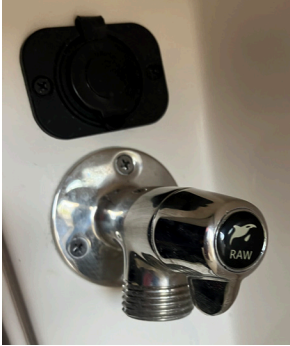
Port raw water washdown tap
