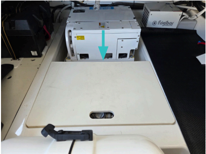
Mid bilge pump
