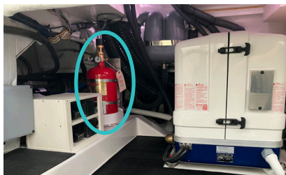
Fixed fire extinguisher
