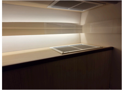
A/C unit vent
