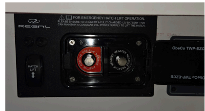
Battery terminals shown
