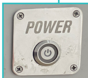
Battery activation panel
