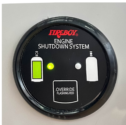
Fireboy shutdown panel
