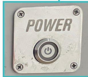
Battery activation panel
