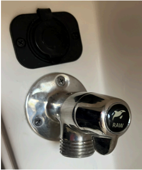
Port raw water washdown tap
