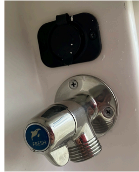
Starboard freshwater washdown tap
