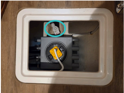
Forward bilge pump
