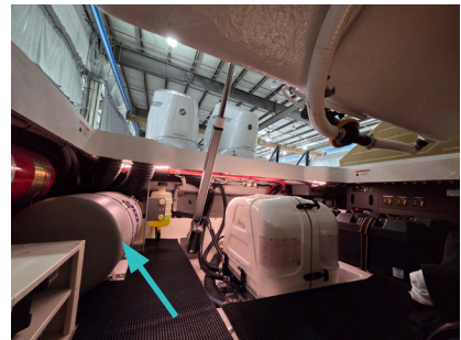
Water heater location
